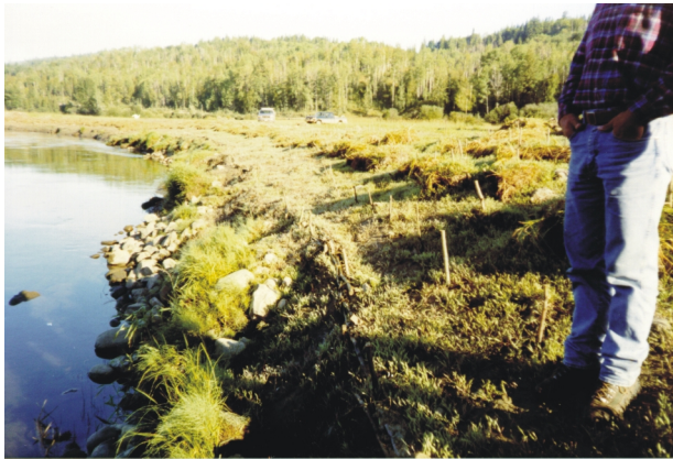
Figure 1: Pull back of vertical banks along the Horsefly River. Note the sods were staked to new slope, willow stakes inserted, horizontal facine at bottom of slope, and initial groundcover with fall rye.
