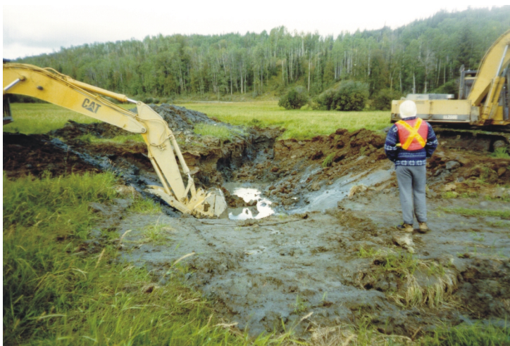
Figure 2: Beginning the excavation of the groundwater channel along depression in floodplain, Horsefly River.
