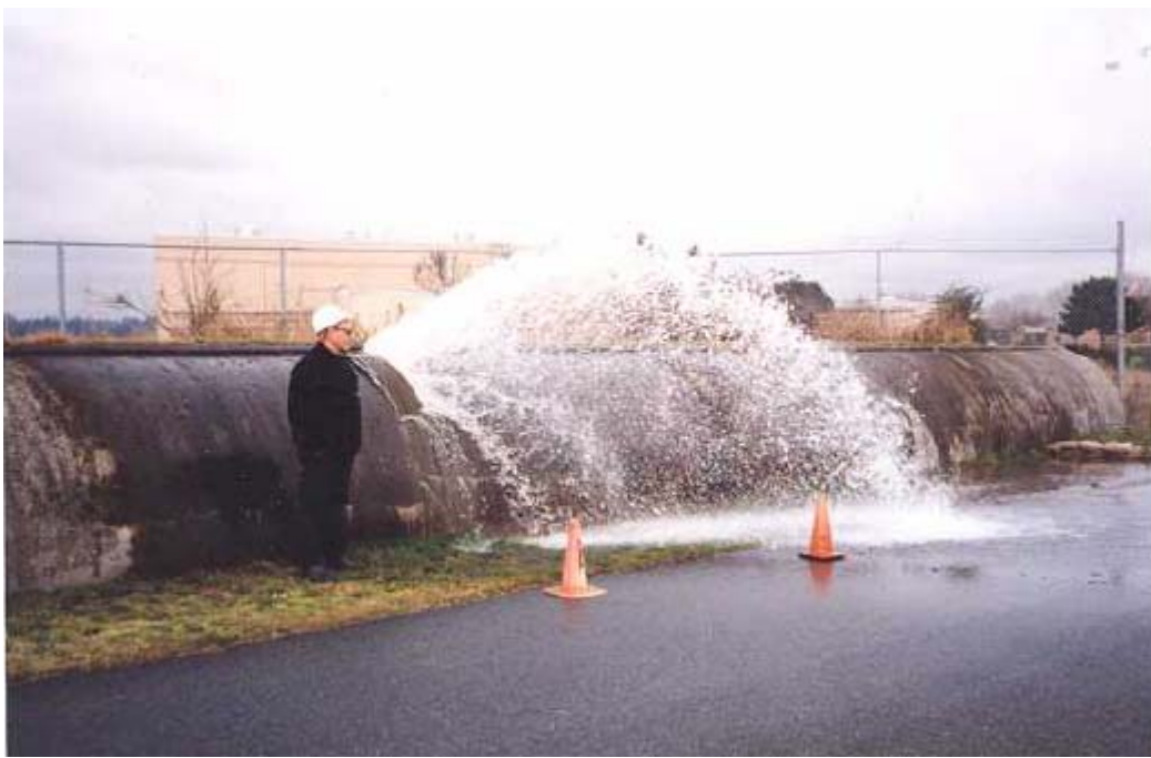
Figure 8: Leak from an effluent outfall conduit at a large wastewater treatment plant (courtesy GVRD).
