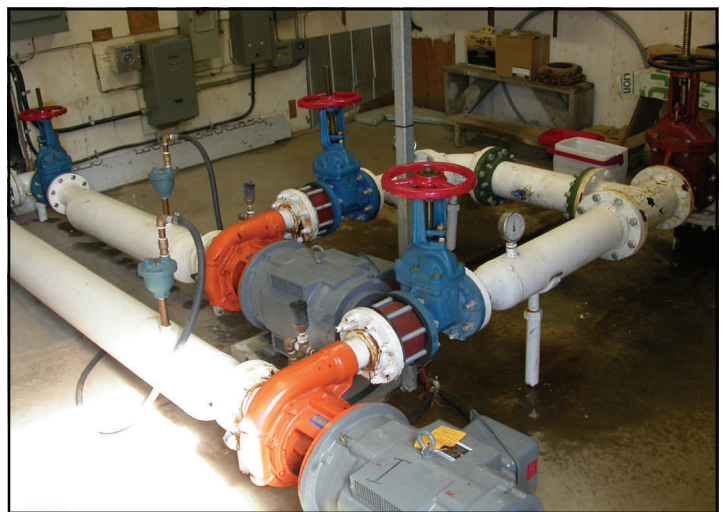
Plate 2. The water piping system inside the Pineview pump house.
