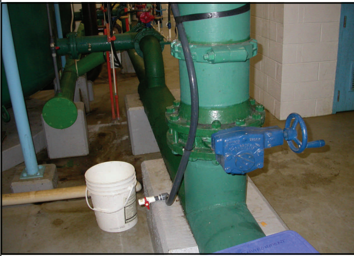
Plate 2. The raw water tap inside the Vanderhoof pump house.
