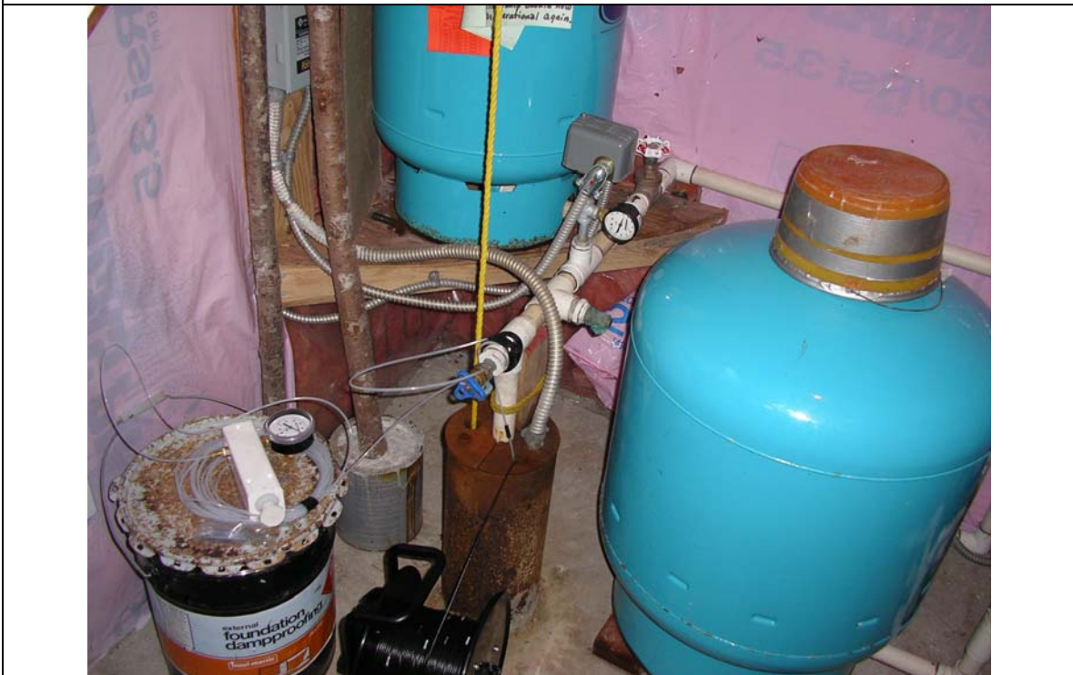
Photo 4. Well 3 with air-line installed and electrical water meter inserted into the front bolt hole.
